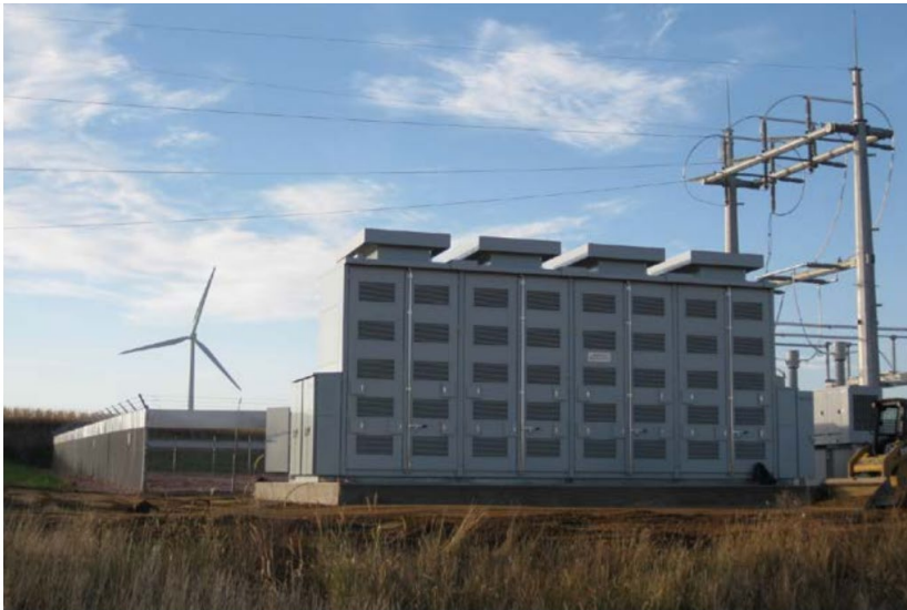
1 MW NAS Battery System installed in Luverne, MN
