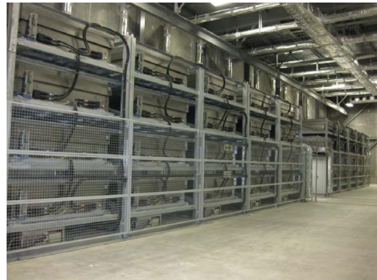
4 MW NAS Battery installation at Presidio, TX
